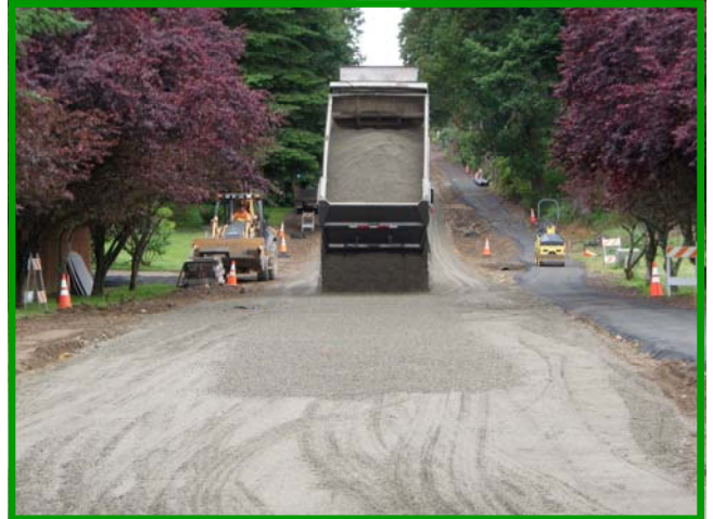
This view of the East Price Street Improvement shows many elements of the project — construction of a new pathway for pedestrians and the newly widened roadway. A truck places gravel in preparation for the new chipsealed surface.
