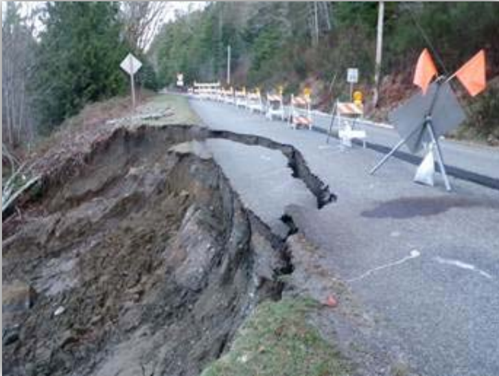
The March 6, 2014, landslide on Dosewallips Road threatened property below the road and access to homes beyond the slide.
