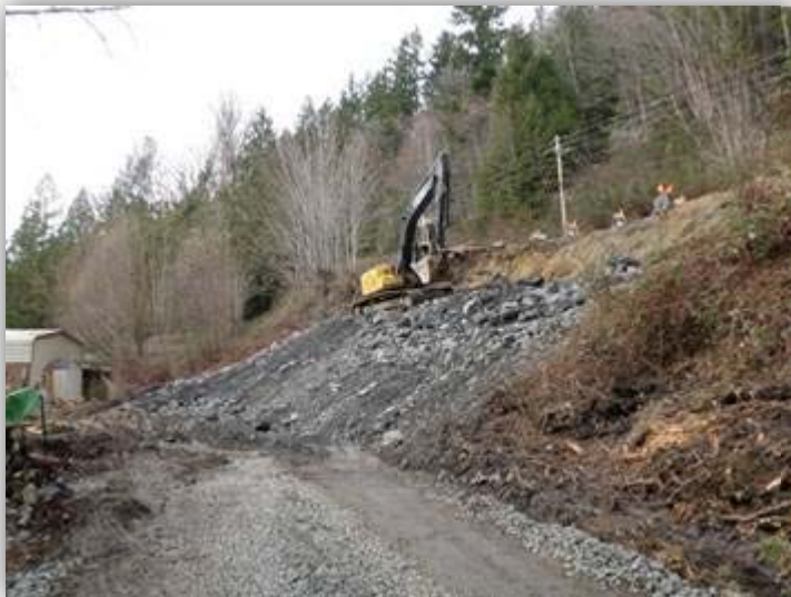
Public Works, with additional trucking from Seton Construction, hauled more than 1,500 yards of mud and debris off the site before slope reconstruction could begin.
