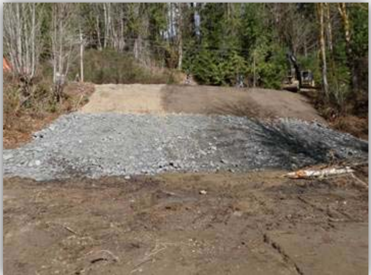
The slope along the road was reconstructed with 2,500 tons of rip rap and other materials. Two-way traffic along Dosewallips Road was restored within two weeks.
