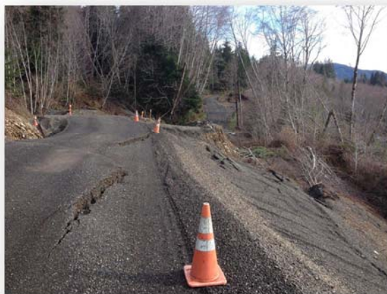
Undie Road Deep-Seated Landslide Damage – February 2016
