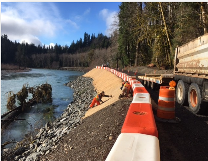
Workers place erosion protection on new slope just before reopening the road.
