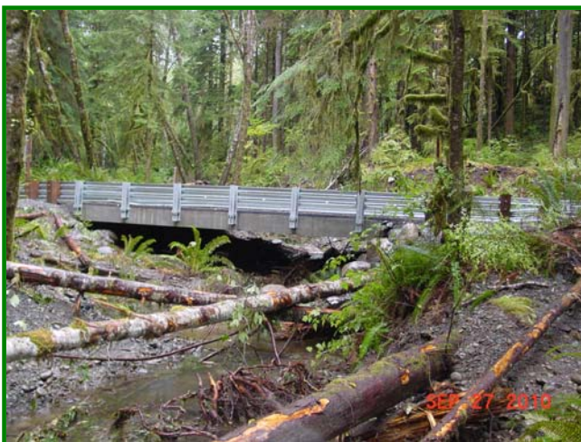
The new Pole Creek culvert is a benefit to both stream habitat . . .
