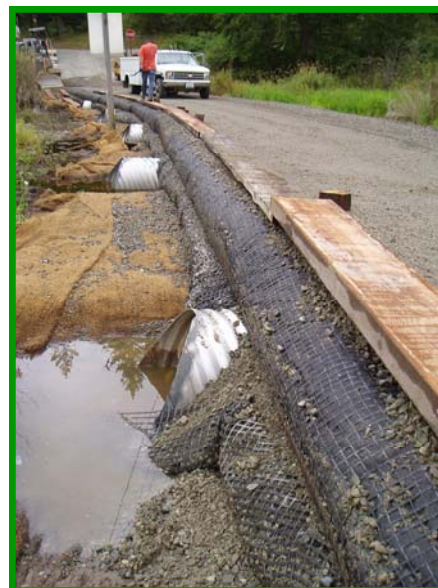
3. Construction included raising the road bed two feet with geogrid wrapped gravel layers to ensure road stability and placing and compacting crushed gravel surfacing.
